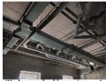
Washroom plumbing system There is water and pipe drain pipe (100mm) and vent pipe (50mm) for foul smell.
