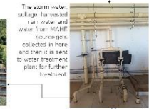
Pump room with generator
