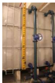
Water Suction Tanks
