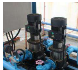
Hydro pneumatic pumps
